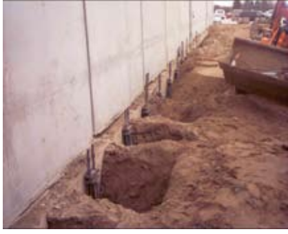
With wall elevation restored and beam straightened, pier holes were filled to final grade.
